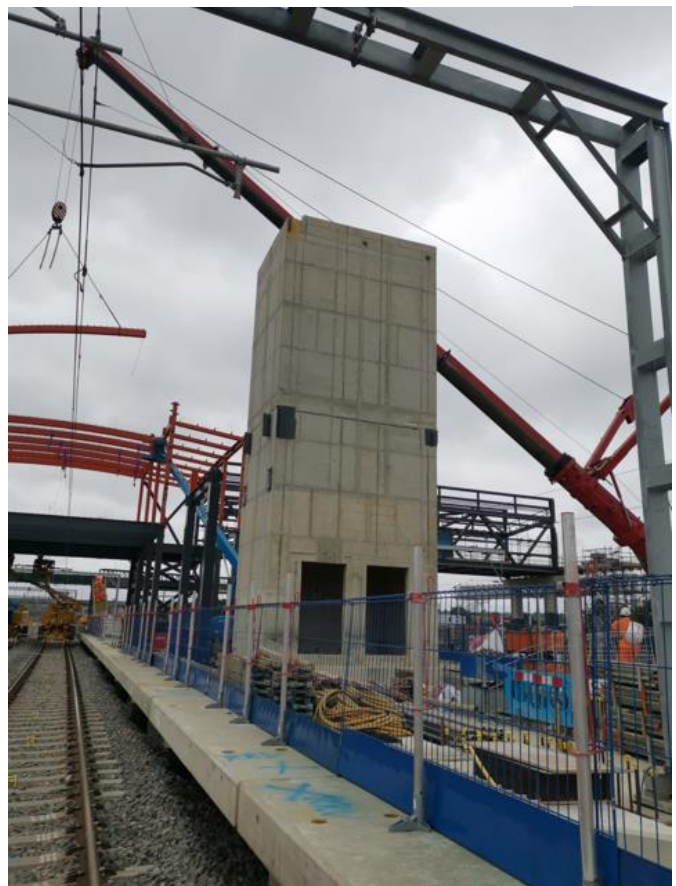
New station lift shaft, with no scaffolding
